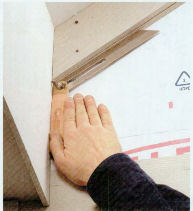
15 Use a T-bevel to determine the angle of the roof line on the gable ends of the house. Transfer the angle to the panels, and cut them to fit.
