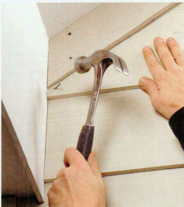
16 Keep the panels \frac{1}{8} " from the rake boards, and nail them in place along the gable end.
