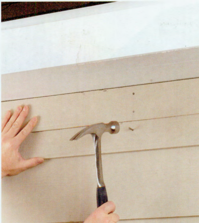
14 Rip the last row of panels to fit \frac{1}{8} " below the frieze boards under the horizontal eaves. Nail the panels in place.
